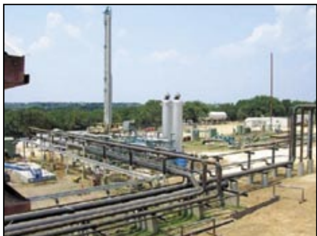
Tolar Plant in Tolar, Tex., updated by Momentum, a subsidiary of Peak, that by year’s end will process up to 40 MMcfd.
